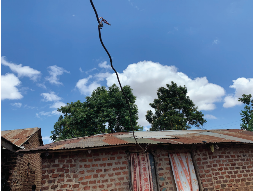
Photo caption: A cable extending into a household to provide electricity, likely as part of a collective metered connection. Photo by Jess Kersey.
