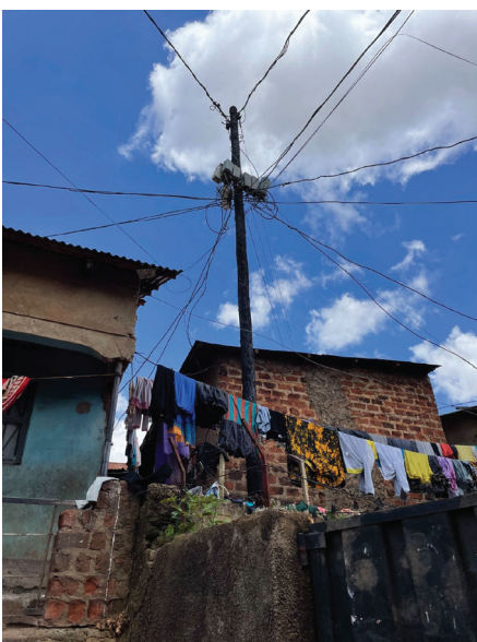
Photo caption: Laundry lines in close proximity to electrical wires and metal roofing. Photo by Elena van Hove.
