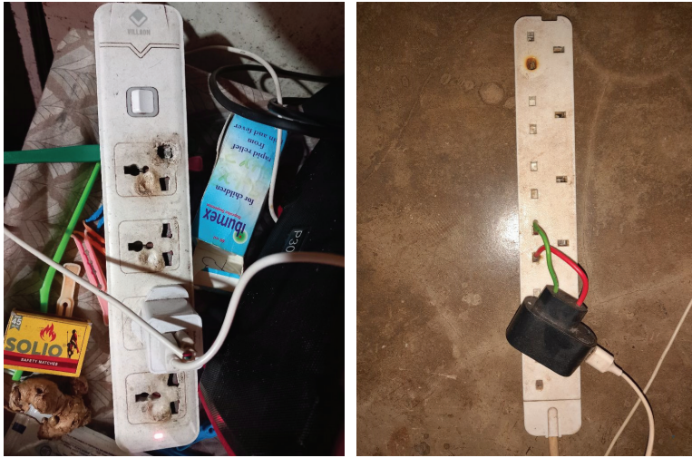
Photo caption: An extension cable in use, burnt in several places from overcurrent (left). A charging block with missing prongs is wired directly into an extension cable (right). Photos by Paul Kyoma.
